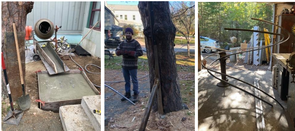
Figure 54. Pouring the concrete pad, installing the support brace, and bending the steel spirals.
