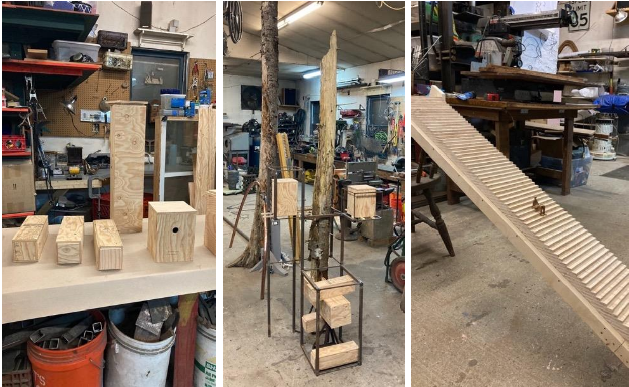
Figure 65. Development of the main structure. (Left) modifies nest boxes will be inserted inside the building and encapsulated in woodcrete for thermal buffering, (center) the steel structure holding the building and the salvaged snag, (right) wooden mold for staircases. Staircases will function as cover objects where they meet the ground, and the space behind the staircases will be designed for use as interstitial space. Source: RJH Artworks, 2022
