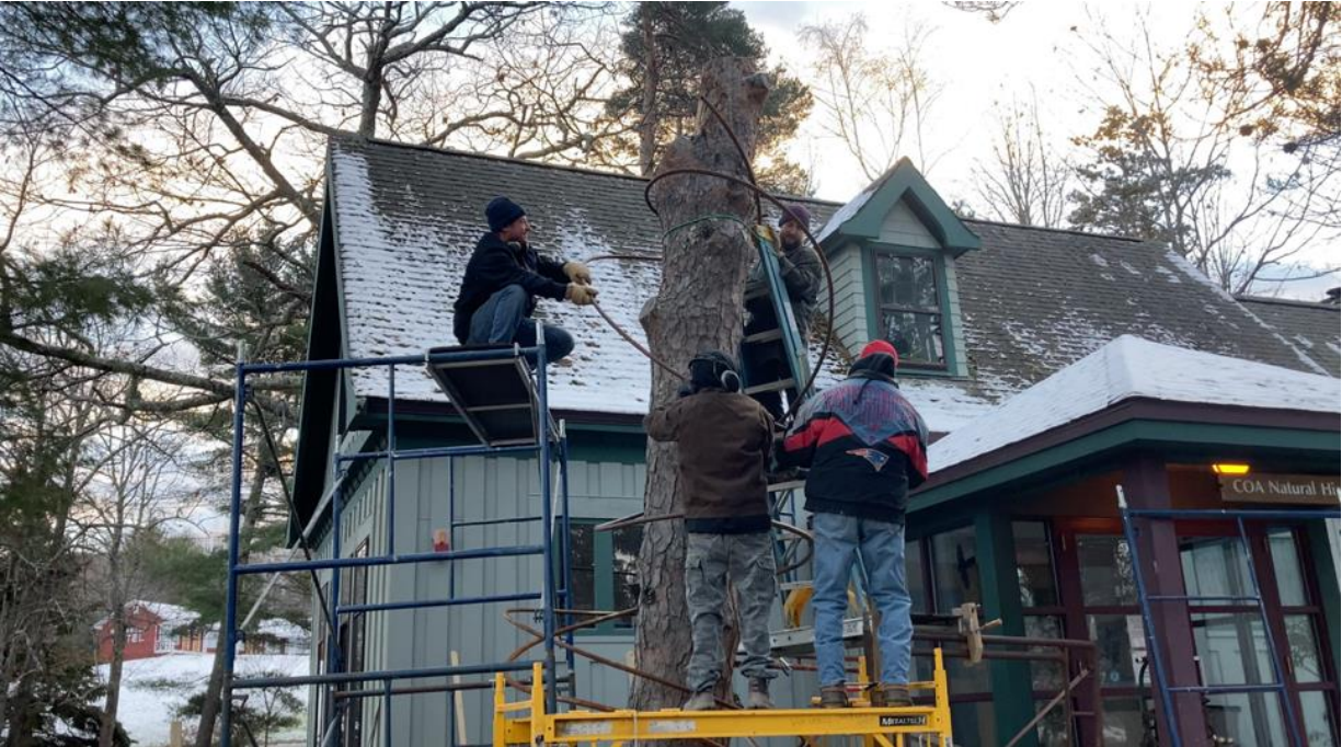
Figure 55. Installing the spirals around the snag with my work crew of volunteers. The spirals were welded to the support base near the bottom and attached to the tree near the top.
